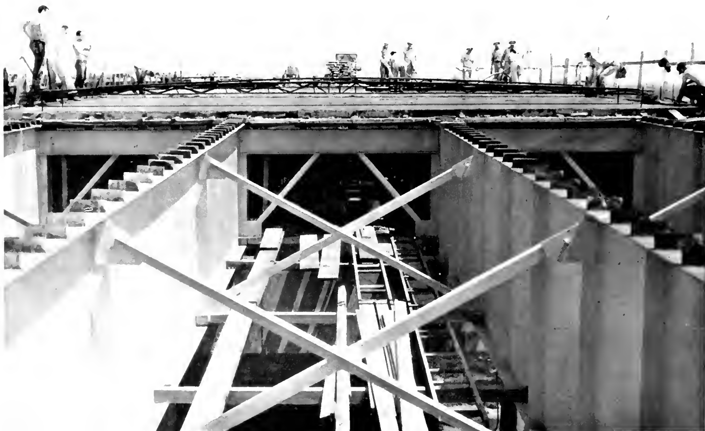
Placing deck slab concrete one span length from east end of Union Pacific Railroad East Yard Overhead
